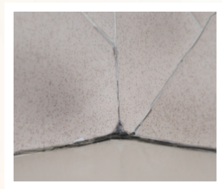
Black Mold Caulking at Tub Deck
